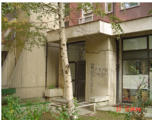
Fig. VIII. Building located over erosion
